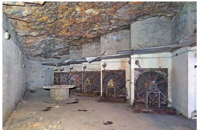
Calpe Hole generating station: a flight of six fan-cooled radiators, set in a diagonal wall across the chamber.
